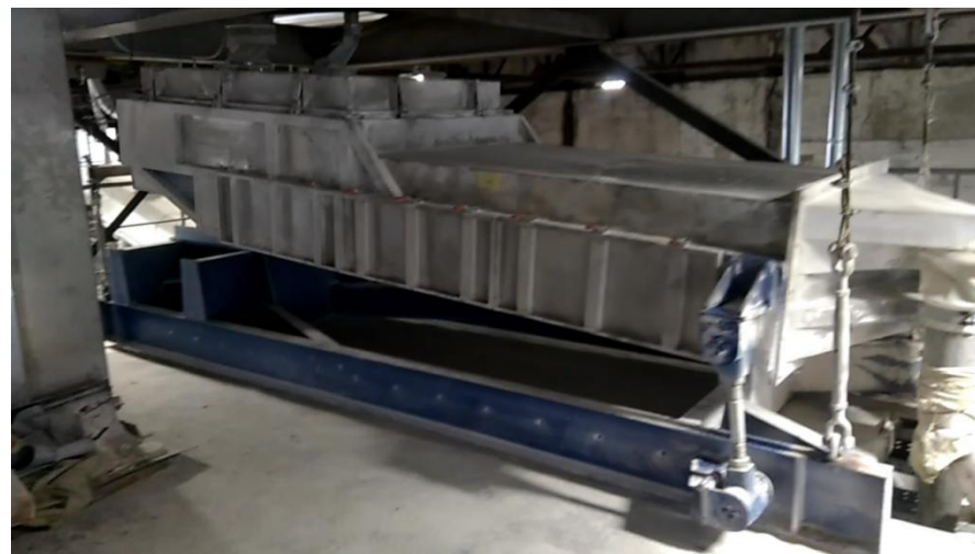
MHG Gyrotary Screen at Sugar Screening site
