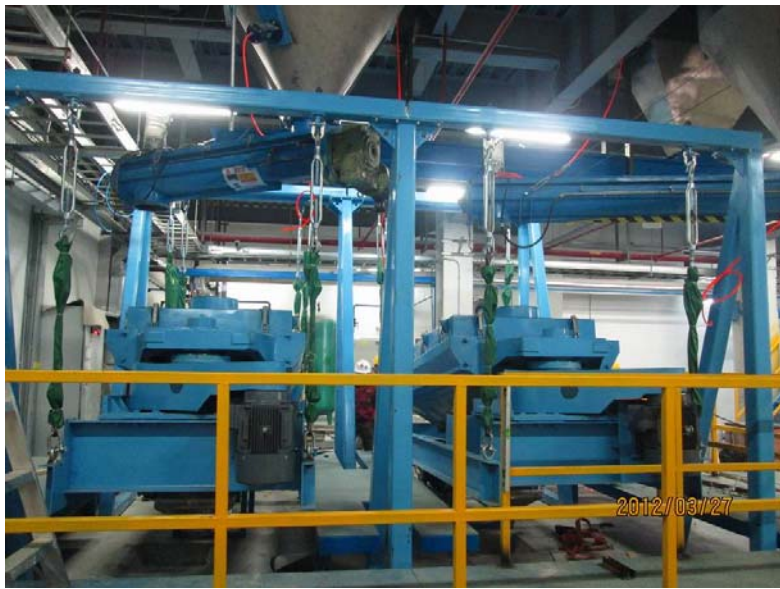
MH Gyratory Screen at PVC screening site
